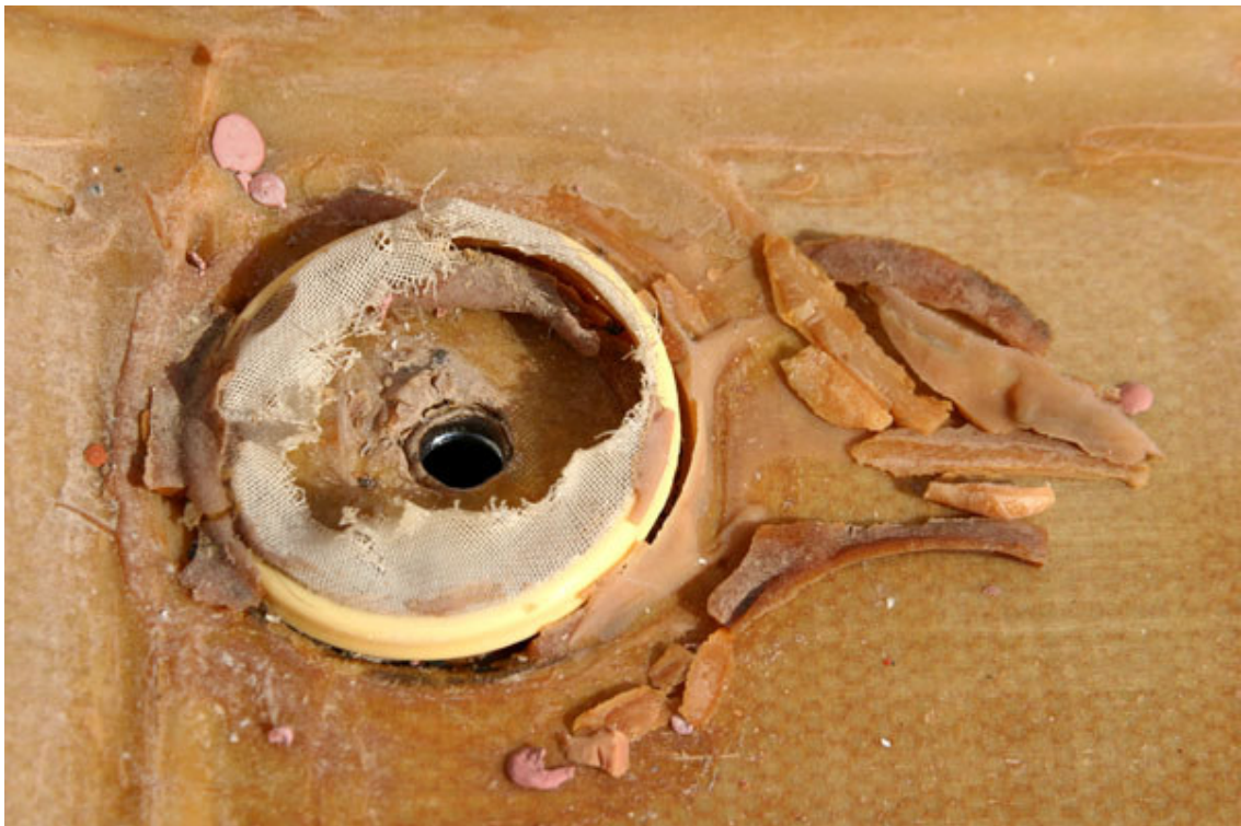
Figure 3: Debris and Strainer Disintegration
