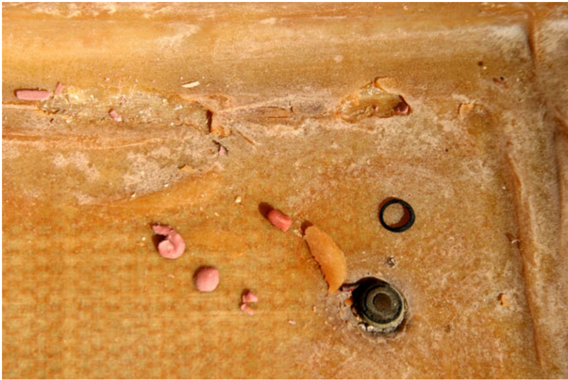
Figure 2: Debris and Deterioration of Edge Joint
