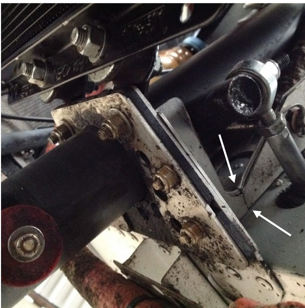
Figure 2.1: cracked support bracket viewed from below (port side of nose leg)
